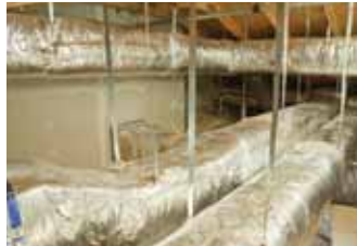
Cottage 6B, Insulated Sheet Metal Ductwork
