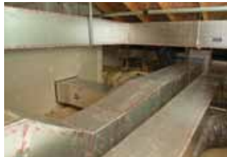
Cottage 6A, The Kingspan KoolDuct™ System
